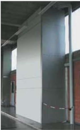
Units installed in a factory
